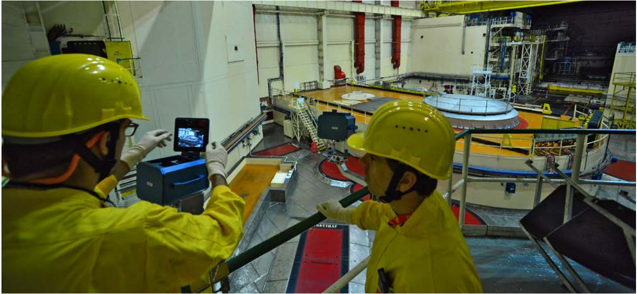
Inspectors installing a video surveillance system to monitor a nuclear power reactor to confirm that any access to the reactor is in agreement with declarations. The light blue object is the reactor cover, which must be removed for access to the reactor fuel. Photo: D. Calma, IAEA.
